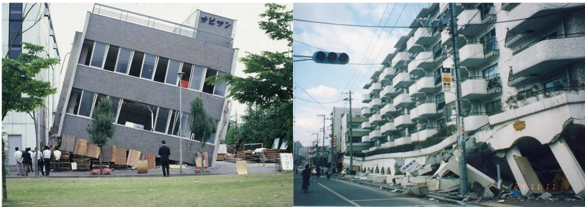
Figure 7. Story collapse of reinforced concrete buildings due to past earthquakes: 1978 Miyagi-ken-oki Earthquake (left), 1995 Kobe Earthquake (right), after [27]
