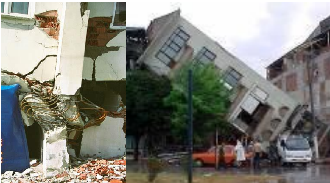
Figure 11. Collapse associated with beam-column joint failure, 1994 Northridge earthquake (left); Foundation failure: Inadequate foundation conditions, including ground failure, ground settlement (right), after [30]
