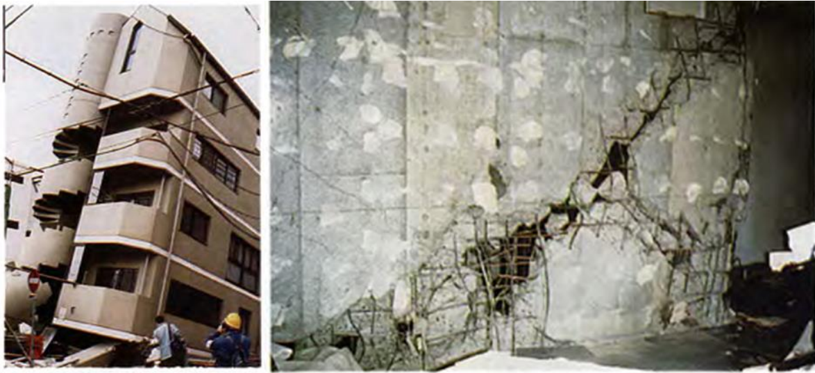
Figure 9. Shear failure of a column due to inadequate transverse reinforcement, after [28]
