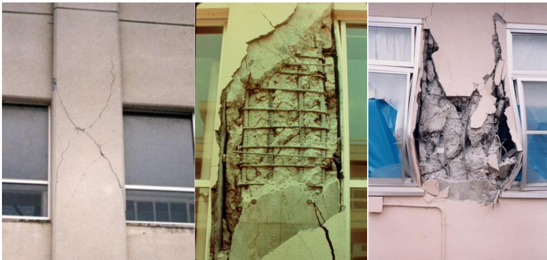
Figure 6. Damage class: III (left), IV (middle) and V (right), after [27]
