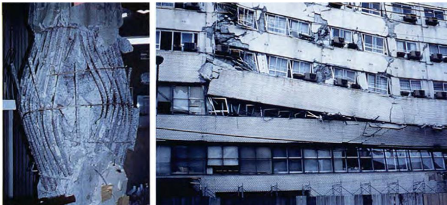
Figure 10. A post-1981 apartment building that collapsed at the soft first story (left) and shear failure of wall (right); An apartment building that collapsed at the third story due to torsion resulting from eccentricities of stiffness and mass (left), after [29]
