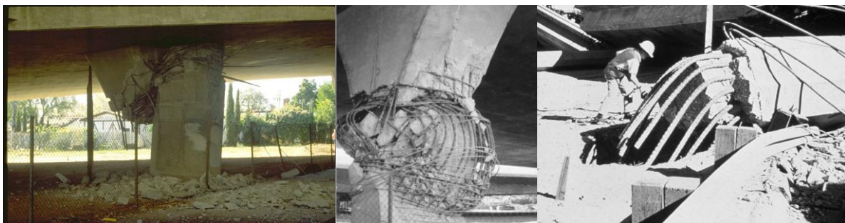
Figure 1. Shear failure, 1971 San Fernando earthquake; RC column failure modes; Compression failure of confined concrete; RC column failure modes Lap-splice failure [19]
