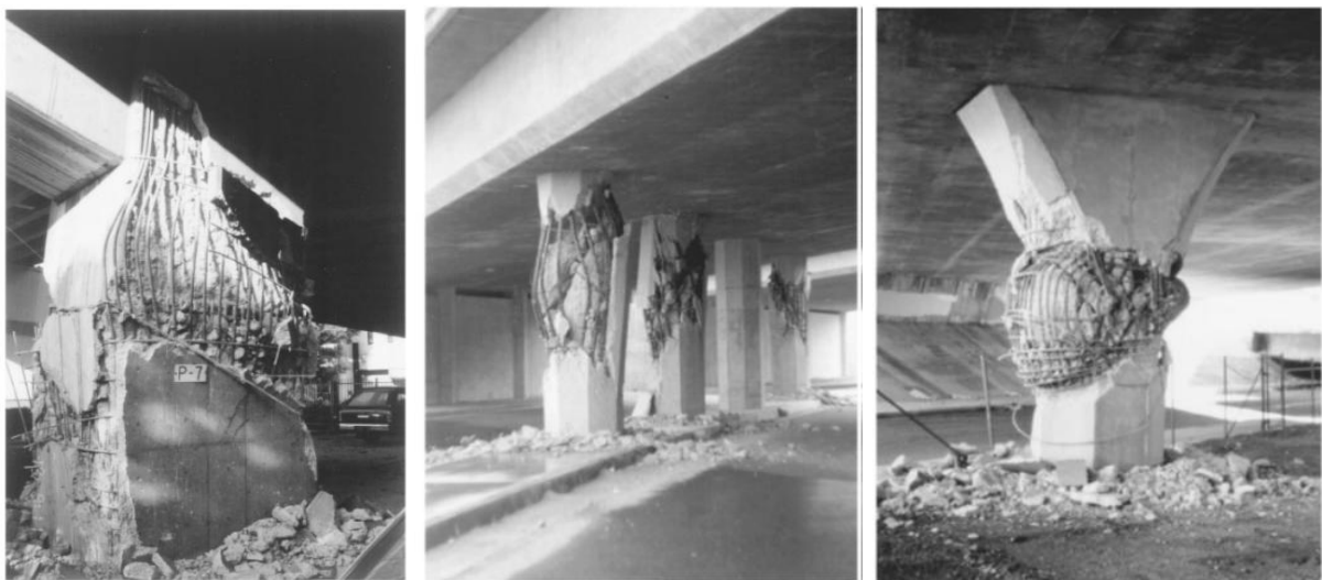
Figure 11. Failure of columns with longitudinal reinforcement cutoffs near midheight in the 1995 Hyogo-Ken Nanbu earthquake after [8]; of the Route 5/210 interchange during the 1971 San Fernando earthquake after [8]; Failure of flared column in the Route 118, Mission-Gothic Undercrossing, in the 1994 Northridge earthquake[11]
