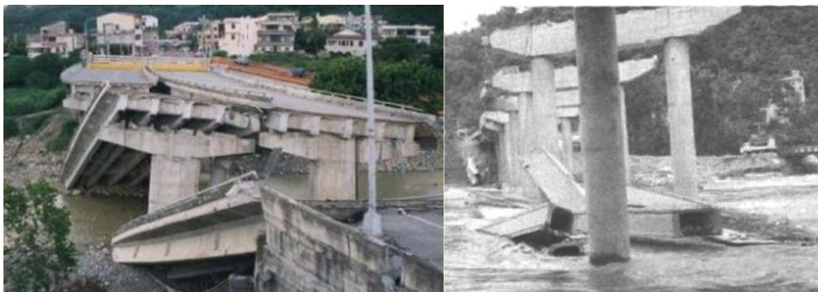
Figure 13. Seismic damage of foundation displacement, after [22]
