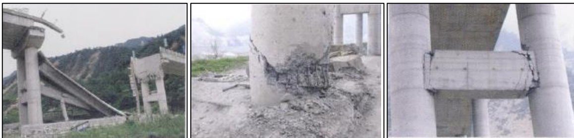
Figure 12. Girders falling of the Gaoyuan Bridge; Piers seismic damage of the Baihua Bridge [22]
