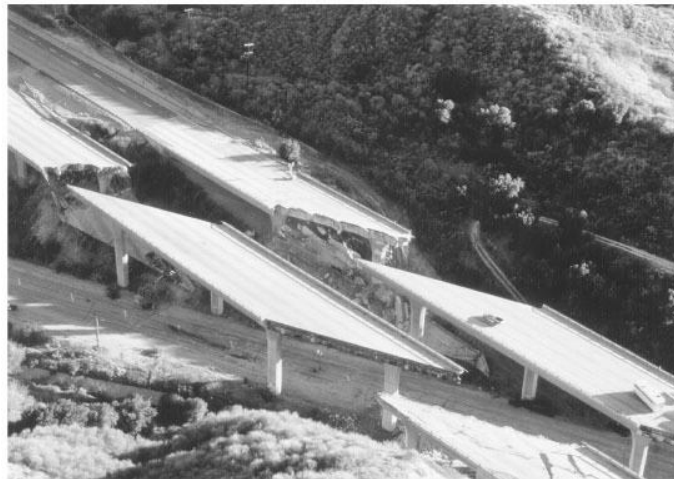
Figure 9. Gavin Canyon Undercrossing collapse in the 1994 Northridge earthquake, after [8]
