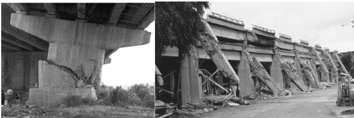
Figure 7. Column shear damage (left), Cypress Street Viaduct collapse in the 1989 Loma Prieta earthquake (right), after [12]
