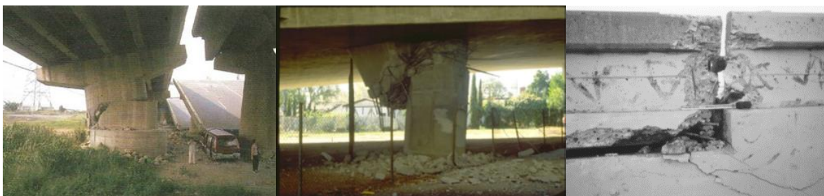
Figure 6. Collapsed spans and damaged piers bridge at the third span, Taiwan 1999, after (Sung et al., 2012), cited in [1], Severe Damage: Shear failure 1971 San Fernando Earthquake, after [16], Santa Clara River Bridge pounding damage in 1994 North-bridge EQ, after [21]
