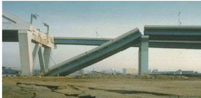
Figure 5. Unseating damage (Kobe, 1995), after [16]
