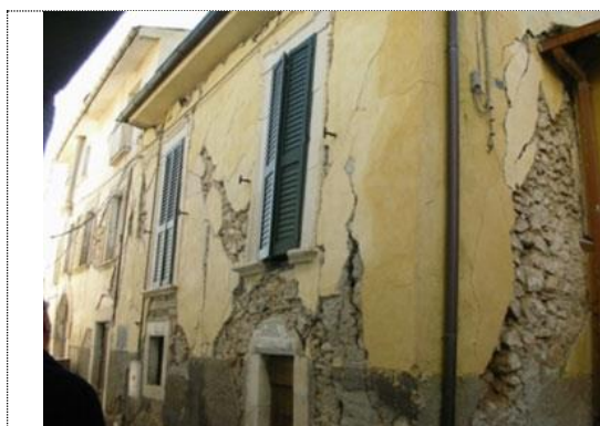
Fig. 11. Severe damages to shear walls and spandrels 2009 Eq. L'Aquila, Italy, [22]
