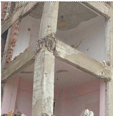
Fig. 5. Beam-column joint damage, Turkey Koceli, 1999, after [17]
