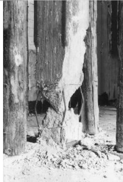
Fig. 4. Column failure due to excessive axial load and insufficient stirrups
