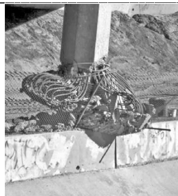
Fig. 6. Bursting failure in a column, Northridge, California, 1994, after [5]
