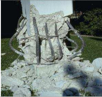
Fig. 1. Poor detail of transversal reinforcement
