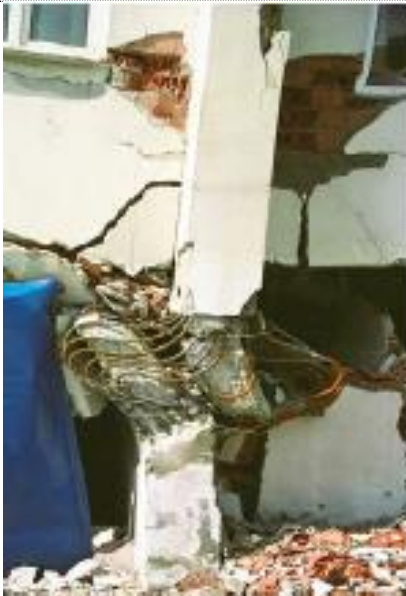
Fig. 3. Collapse with column shear and axial failure. Koceali Eq. 1999.
