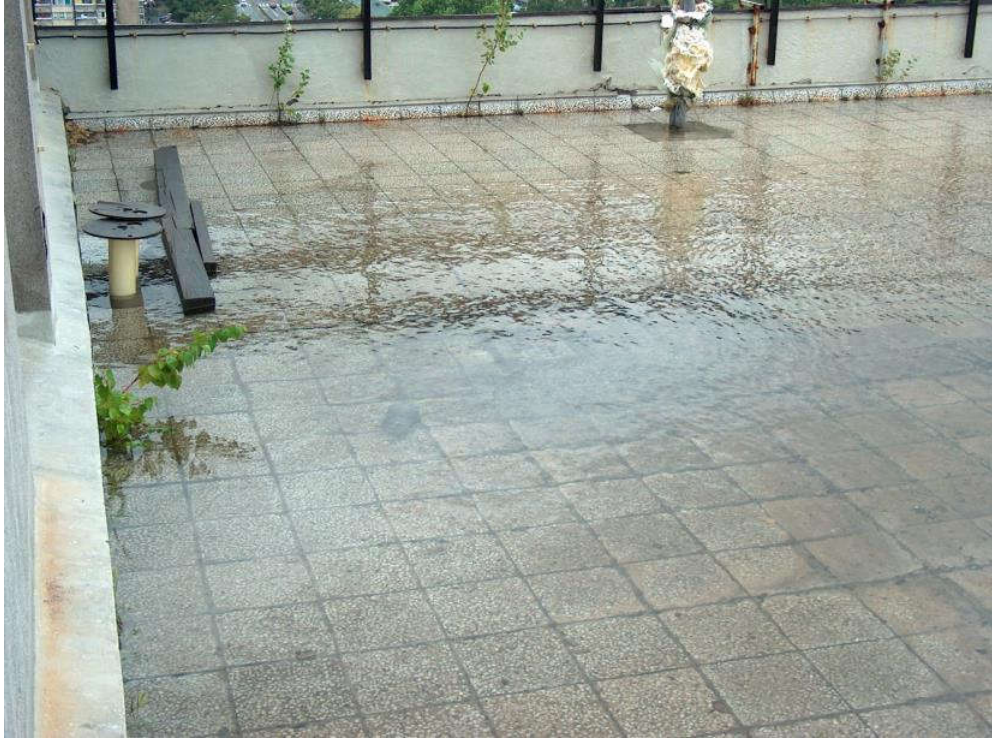
Figure 5. A view of the flooded roof terrace and unplanned roof plants near the attics. July 2004.
