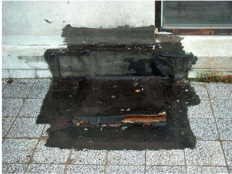
Figure 7. Opening on the roof closed off with the plywood panel. Waterproofing damaged in one part. July 2004.
