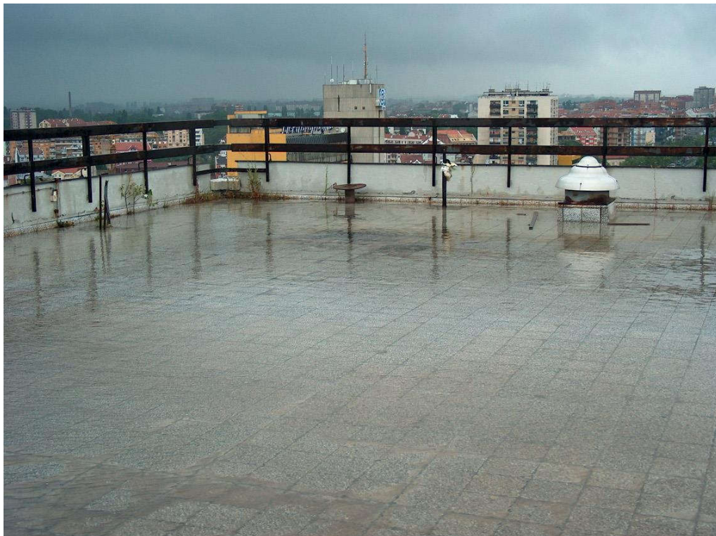
Figure 6. A view of the flooded roof terrace and unplanned roof plants near the attics. July 2004.
