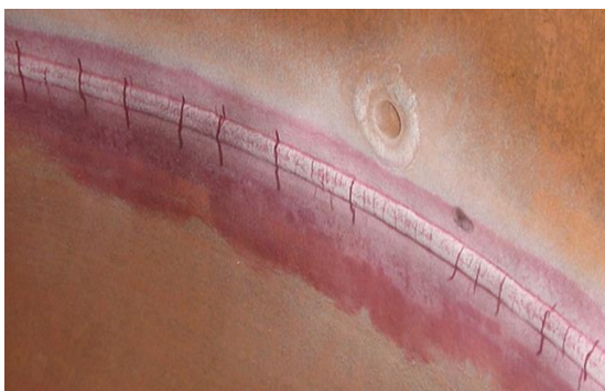
Figure 2. Transversal cracks in the circumferential welded joint.
