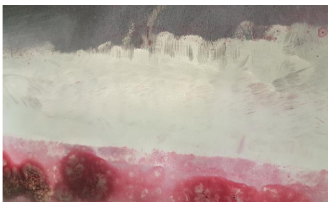
Figure 8. Condition of the circular welded joint after grinding and crack removal.
