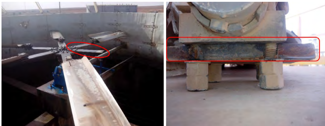
Figure 4 Broken blade at blade holder joint at threaded joints (upper holder split due to fatigue cracks)
