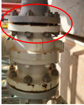
Fig. 2 The flange at the lower nozzle F1 (4") was found distorted, but leaking has not been observed while the vessel was in service
