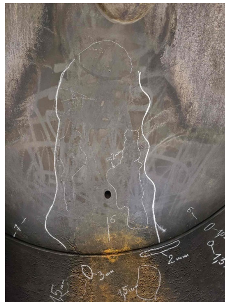
Fig. 4. Left head - close up view on the corroded surface (whole elliptical head has been scanned and minimum thickness was found to be 10.43 mm)
