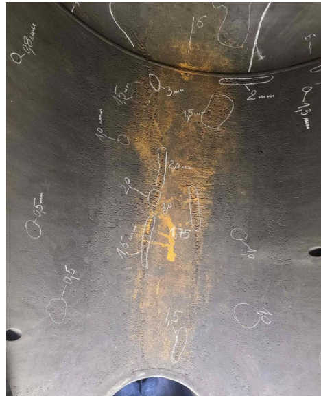
Fig.3. Pitting corrosion has been observed on the lower part of the shell (from 5 to 7 o'clock position) - majority of the pits are between 1.5 to 2.0 mm deep
