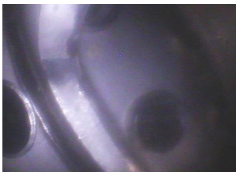
Figure 3. Interior of the header was found in good condition in time of inspection
