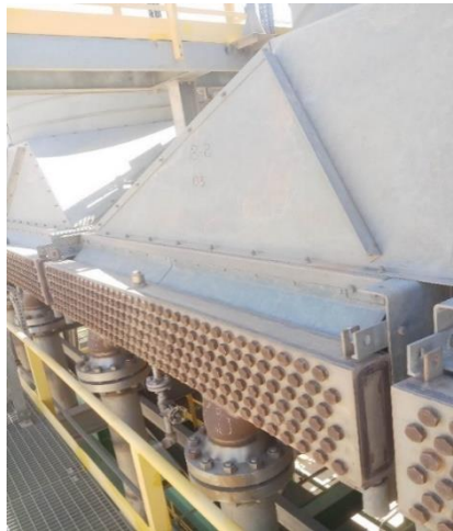
Figure 2. Air cooled heat exchanger (view from the back side)
