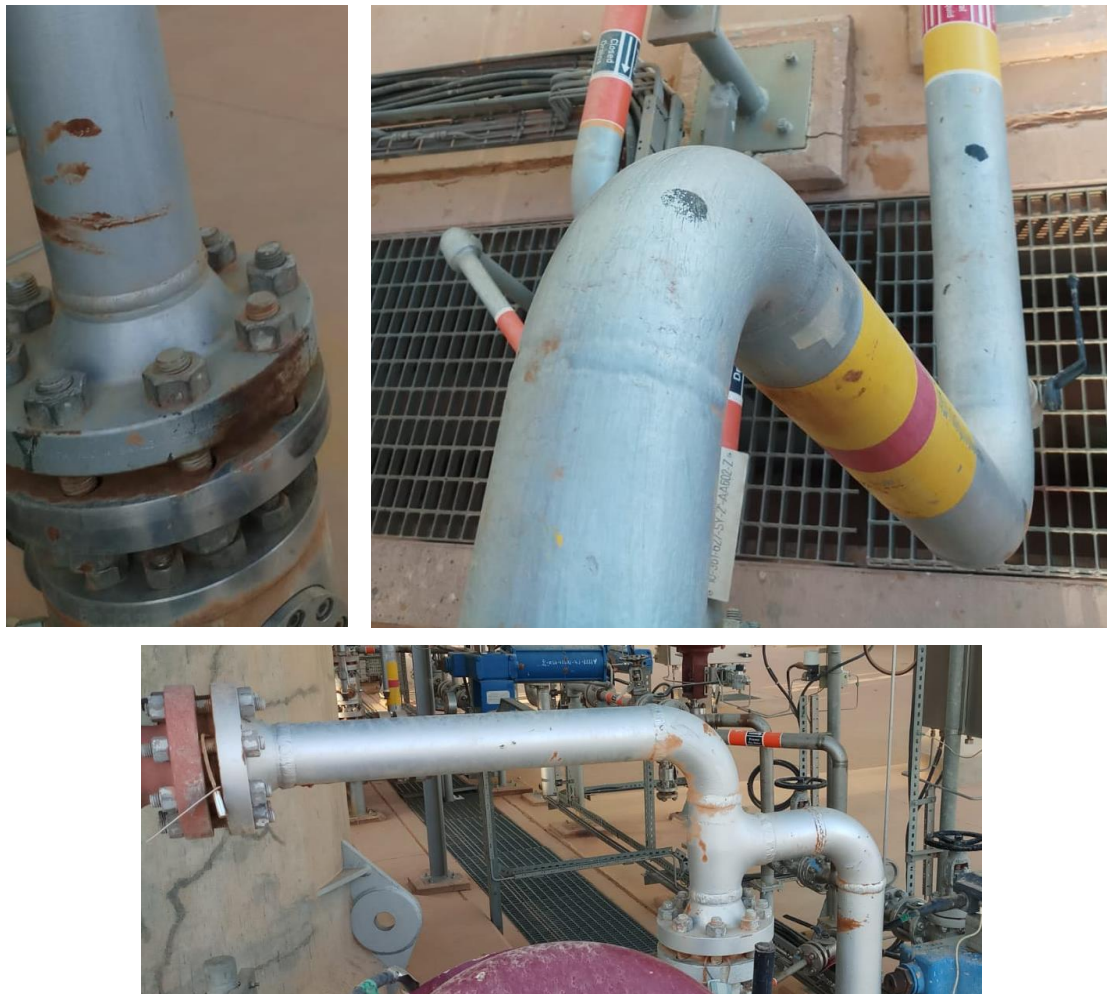
Figure 3. Visual testing of external sides of the pipeline. Pipelines are in good condition.
