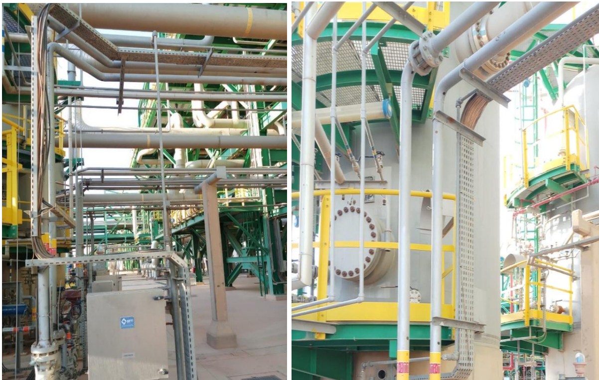
Figure 2. Pipelines at the oil platform
