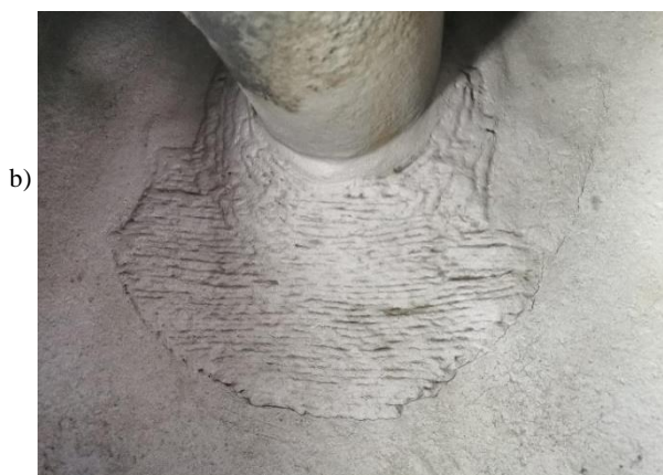
Figure 1. Most common damages in containers: a) wall thinning in the upper mantle and lid; b) cracks in the shower connector areas.
