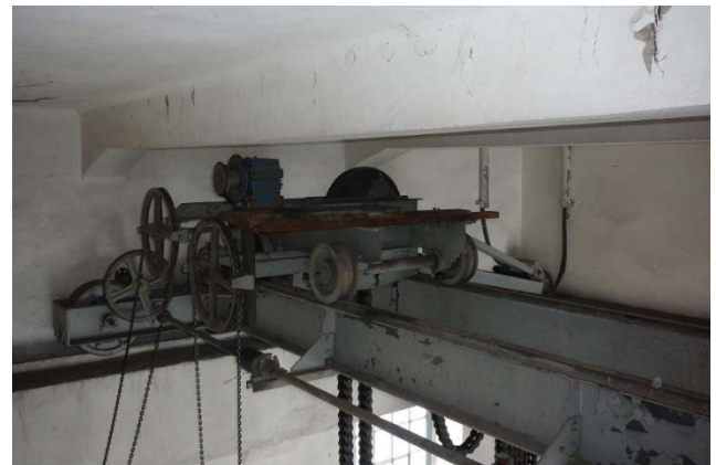
Figure 1: Picture of old crane trolley
