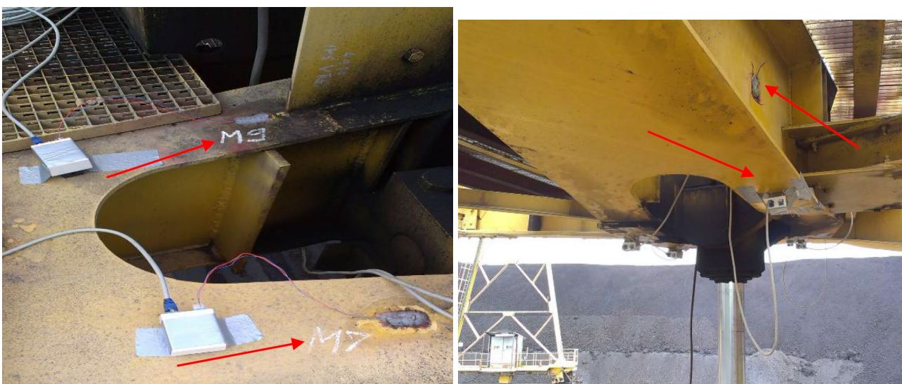
Figure 6. Measurement locations at the vital structure in the area of the cylinder which enables the movement of the bucket-wheel boom
