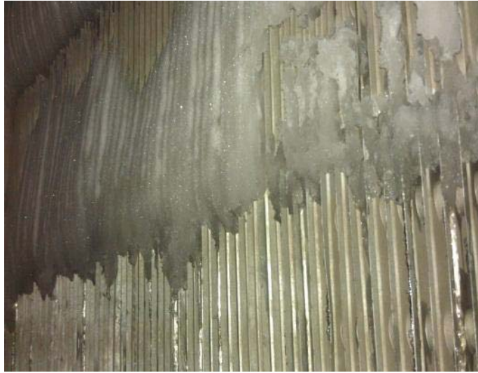
Picture 4. – Evaporator with manually forced defrost iced up (or due to wrong timing of automatic defrosting)
