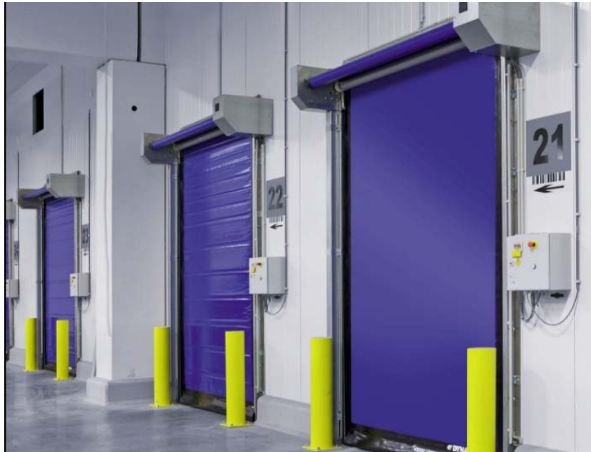
Picture 3. – Cold store doors with automatic mechanisms
