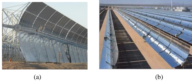
Figure 1: (a) Parabolic trough collector and receiver tube and (b) Field of PTC in work
