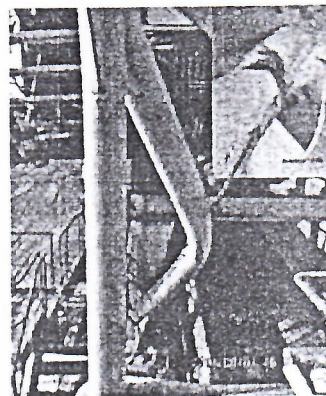
b) Appearance of a part of the damaged vital steel structure
