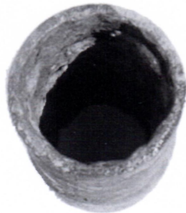
Figure 1. Common corrosion of pipes
