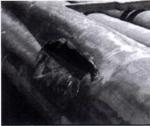
Figure 2. Fracture of the pipes
