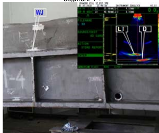
Figure 2. Appearance of segment 4-1 of the upper ring of guide vane apparatus
