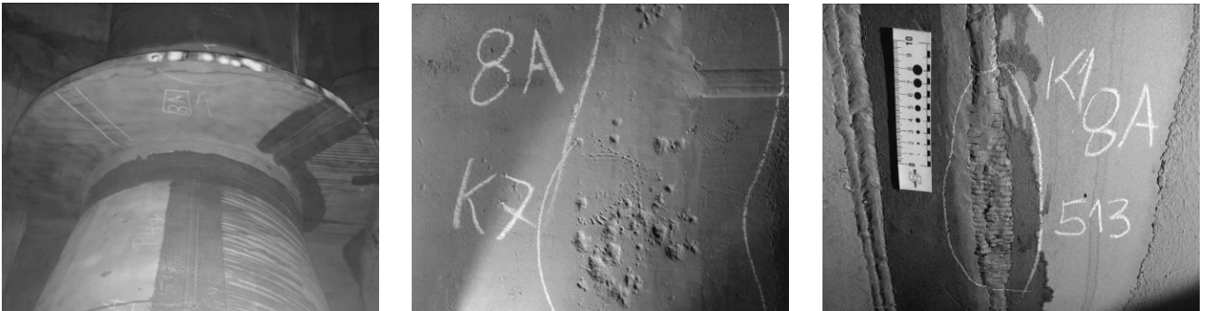
a) Characteristic damages that occur at parent material of the collar and the anchor
