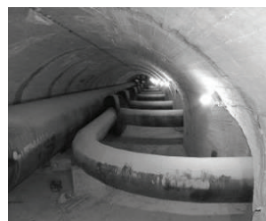
Figure 4. Appearance of the pipeline III with breeches pipes
