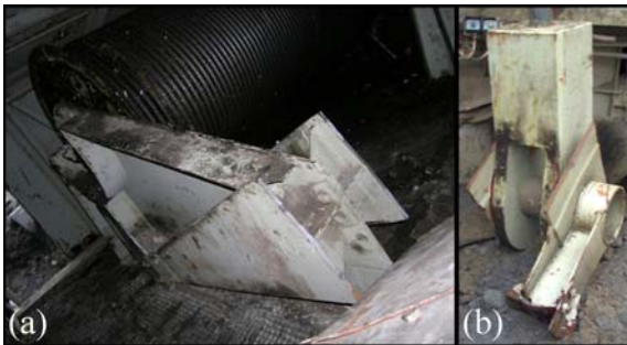
Figure 4: Broken-down support of the right portal tie-rod: (a) element on the counterweight arm and (b) broken-away part.
