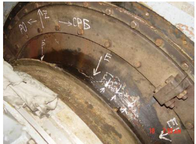
Fig. 2. General appearance of the cracked zone
