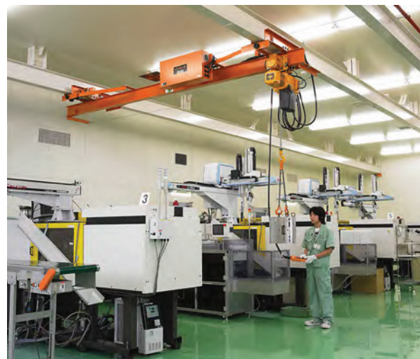
Figure 2. Underhang crane with runway
