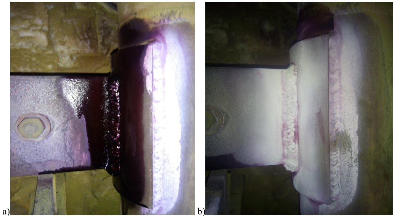
Fig. 3. Crack on support of pipe removed by grinding and repaired by welding, penetrant test was conducted after repair welding and cracks was not found at time of inspection
