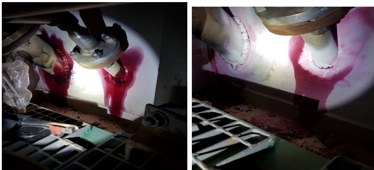
Fig. 4. Cracks on thermocouples removed by grinding and repaired by welding, penetrant test was conducted after repair welding and cracks was not found at time of inspection
