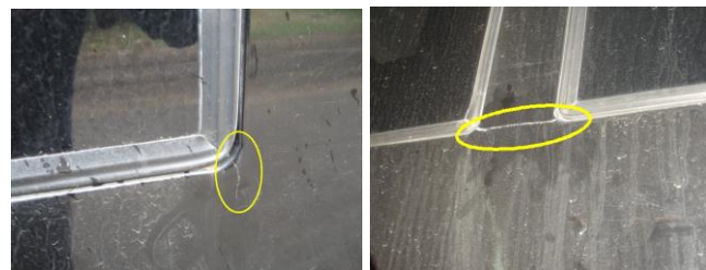
Fig.4. Cracks along window welds
