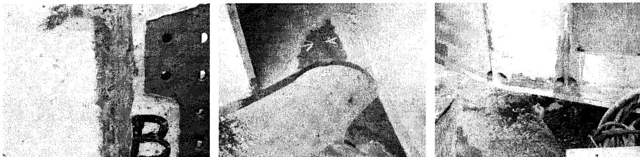
Slika 12. Oštećenja veznih nosača donje gradnje transportnog bagera Figure 12. Damaged connection beams in the excavator lower assembly.
