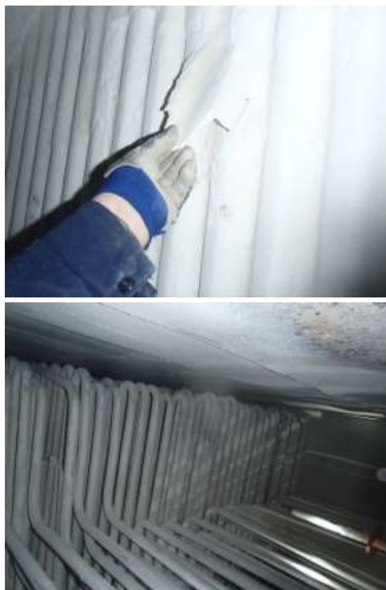
Figure 5 - Interior of flue gas duct. a) Fouling layer on pipes aligned vertically on furnace rear wall; b) Pipe bundles of 1. stage economizer
