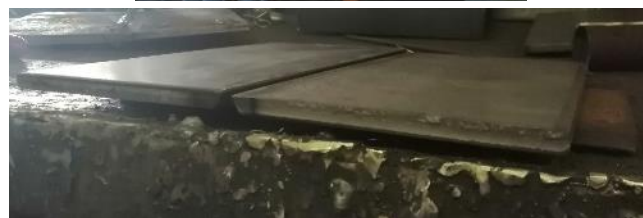
Figure 1. Kemppi Arc Q device used for monitoring of welding parameters (top), and S235JR plates with misalignment being prepared for welding (bottom).
