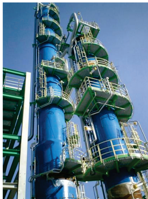
Figure 2. Gas rectification columns
