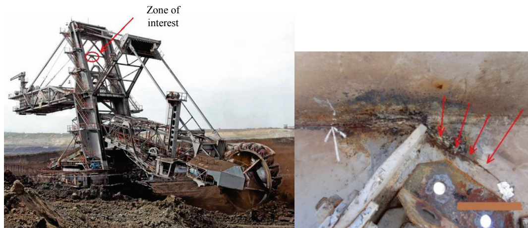
Figure 1 Bucket wheel excavator SchRs630, gusset plate crack position and appearance
