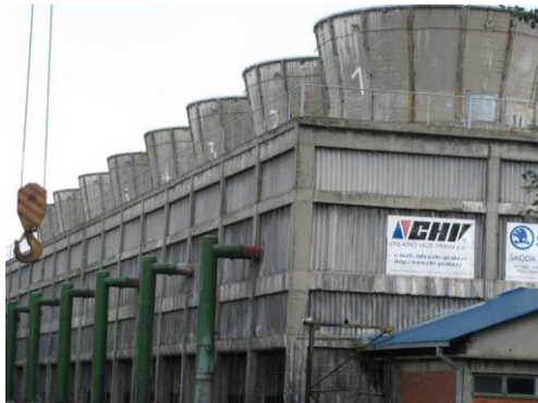
Figure 4. Cooling towers of the power plant
