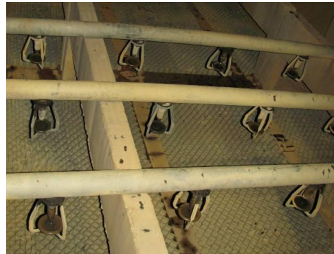
Figure 5. Nozzles and fill packing
