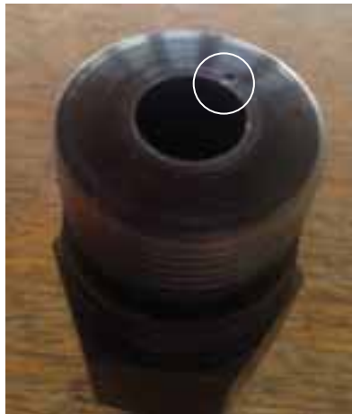
Figure 7. A recess of approximately 1.5 mm in diameter on the front surface of the release valve assembly
