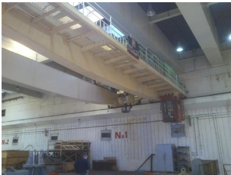
Figure 1. Selected crane in Serbian SME machine hall
