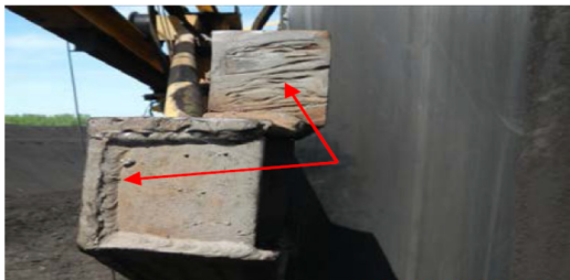
c) Detail that indicates the cause of geodesic deviation of parent material during the repair of carrying structure;
