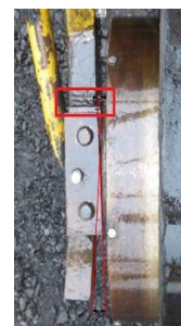
b) Badly executed welded joint and repair carried out in the area of the damage that occurred at the carrying structure of the stacker conveyor rejecting drum
