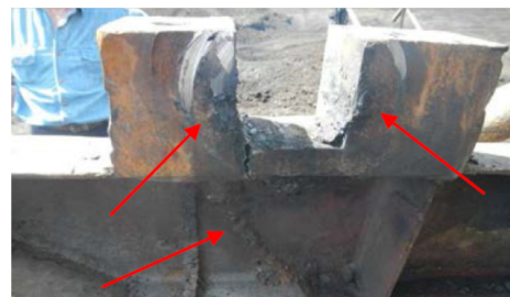
f) Damage and a crack at the carrying structure of an embedding of the stacker conveyor rejecting drum
