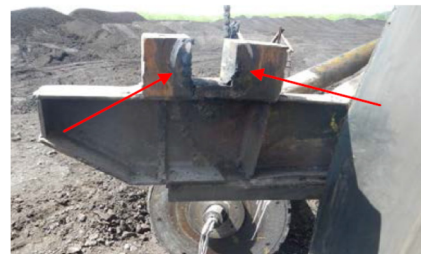
d) Damage at the structure of an embedding of the stacker conveyor rejecting drum – detail;
