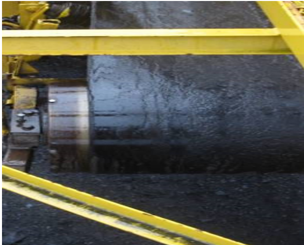
Figure 6. Appearance of the rejecting drum after the installation of new components at the carrying structure
