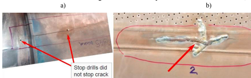
Fig. 4. (a) Crack propagation; (b) First repair: welding of single cracks
