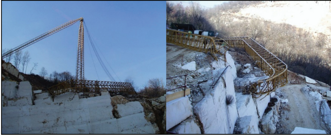
Figure 2: The collapsed boom of the derrick crane
