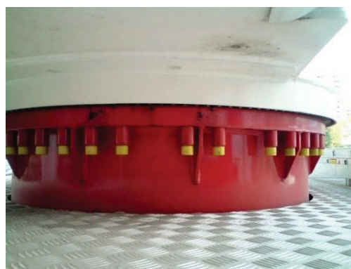
Figure 2 Problematic bolted joint
