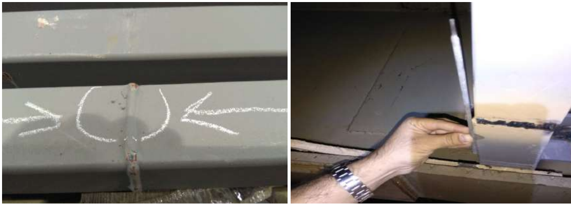
Fig. 4. Irregularity in the butt-welded joint (excess weld metal on the face of the weld)
