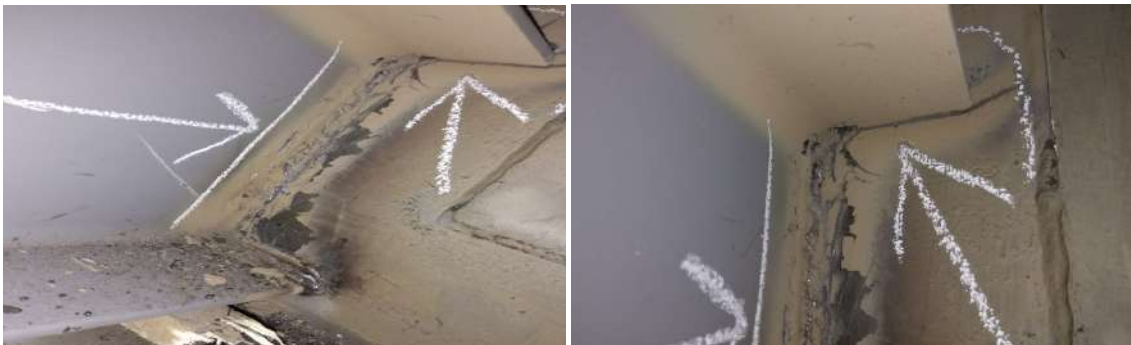
Fig. 5. Irregularity in the welded joint (insufficiently filled grooves)
