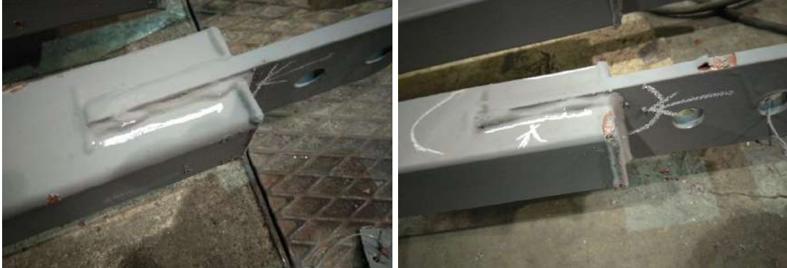
Fig. 3. Irregularity in the butt-welded joint (uneven width of the weld)
